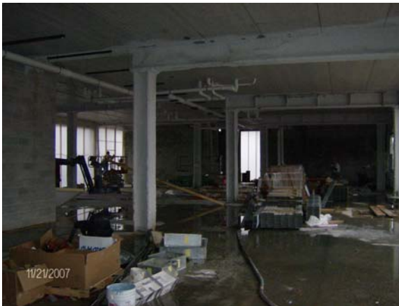
Hotel 1 st Floor Plumbing
